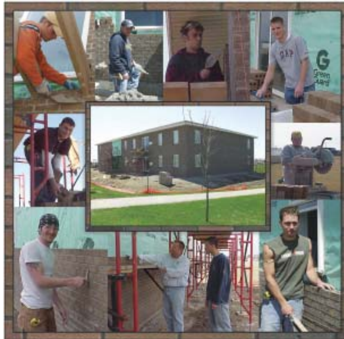
Among the 13 students laying brick at the Foundation’s housing project are (clockwise from upper left corner) Paul Wiegel, Argyle; Jason Welsh, Highland; Tim Otto, Richland Center; Dan Mau, South Wayne; James McKillip, Wauzeka; Andrew Nelson, Fennimore; Shane Tomas, Livingston, with Instructor Don Borchert; Jeremy Reddell, Dodgeville; and Jeff Huehne, Platteville. Students not pictured are Dustin Freymiller, Fennimore; Preston Quinn, Fennimore; Kyle Spensley, Belmont; and Joshua Copsey, Prairie du Chien.
